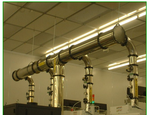
▲ Exhaust ducts separate waste gases by type and protect employees from exposure
