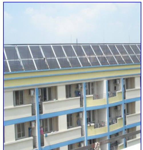
▲ Solar-thermal water heaters on top of the employee dormitory in Shanghai
