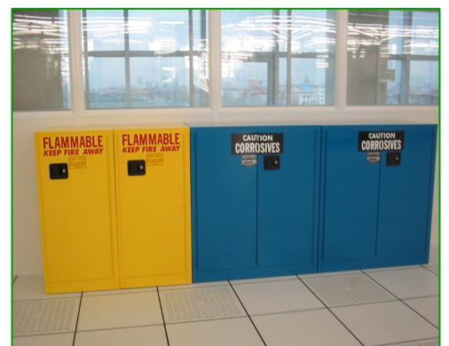
▲ Chemical storage cabinets ensure proper chemical segregation and protection
